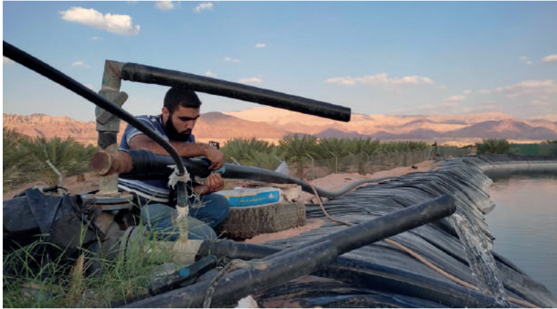
Example of a Flowless hardware installation. (photo: Flowless)
