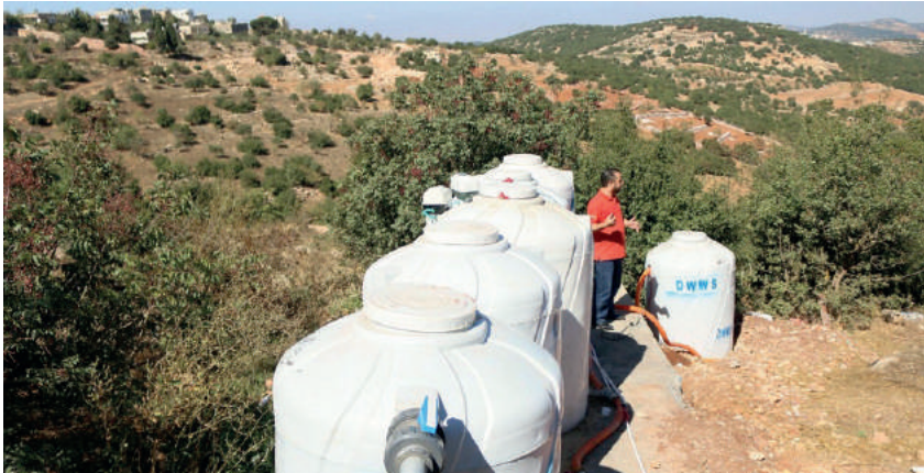
SOLVillion's decentralized wastewater treatment system (photo: SOLVillion)
